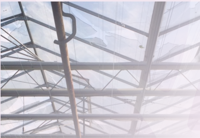
Broken glass at the top of the greenhouse
